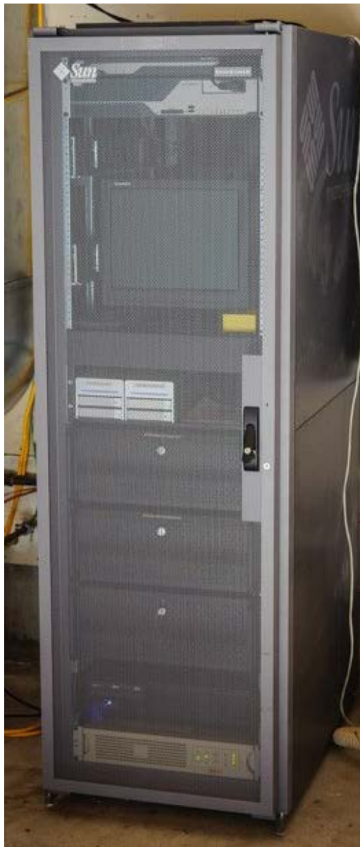
Pops.net server rack in our warehouse.
